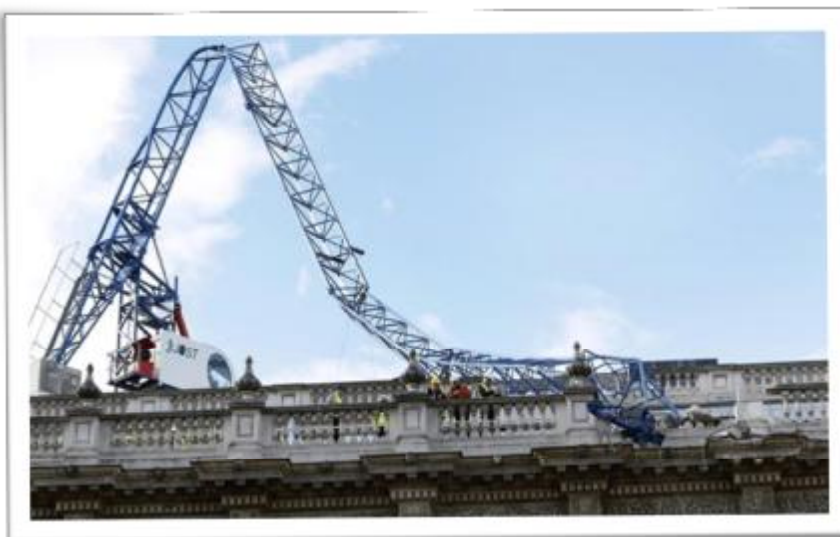
Crane brought down by high winds on the roof of Cabinet Office, Whitehall, 28/10/2013 (AP Photo/Kirsty Wigglesworth).
